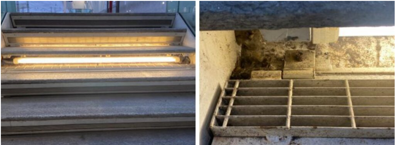
a) Steps of a track access staircase. b) Detail of the riser of a step with an open grid for maintenance (photo credits Augusto Giuffredi).
