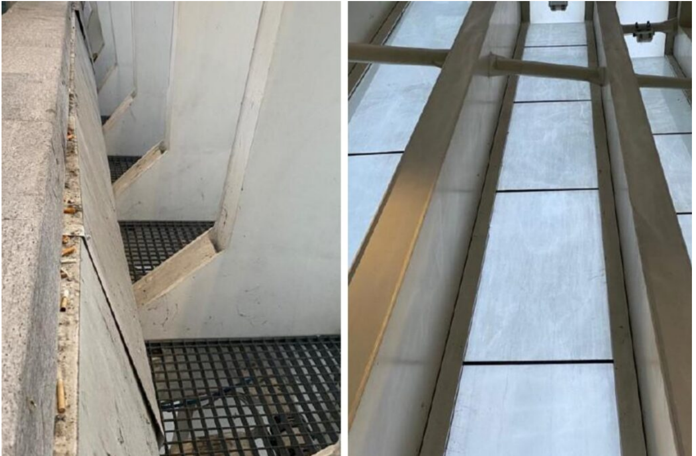
a) Joint between parapet and metal ribs at the height of the boarding sidewalk. b) A section of the ascending glazing with the usual deposit of dust and smog (photo credits Augusto Giuffredi).
