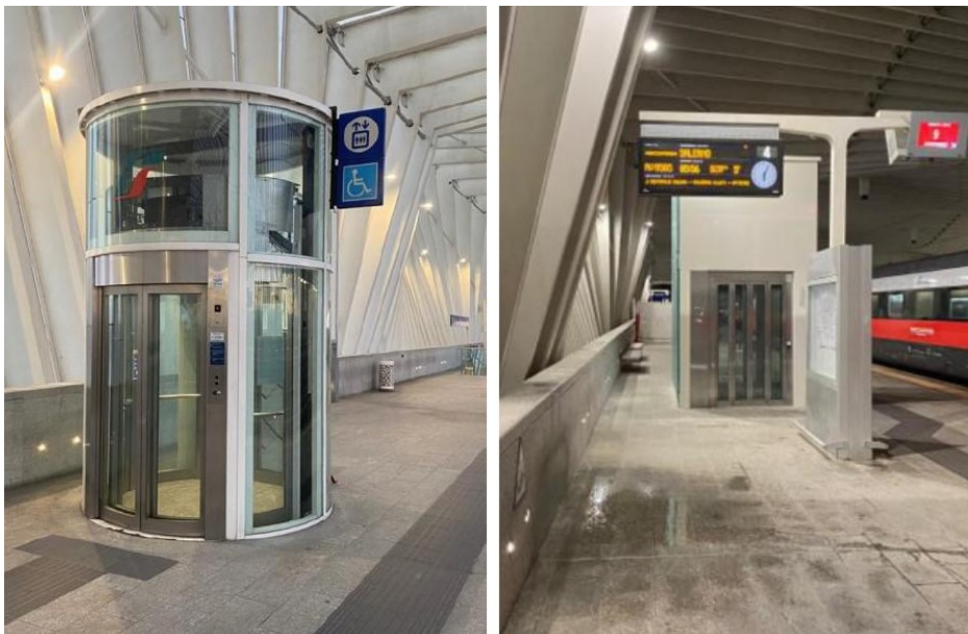
a) One of the two lifts currently in operation, b) one of the new compliant lifts, not yet in operation, photographed at track level (photo credits Augusto Giuffredi).
